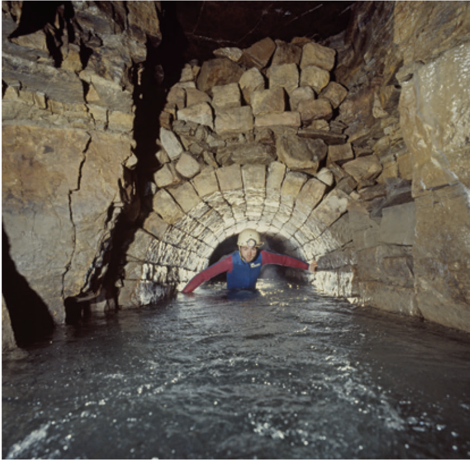
Figure 5. Stone arching to support a section of bad roof in Meerbrook Sough (photo by Paul Deakin). From Trevor D Ford and Jim Rieuwerts, 'Lead Miners' Soughs in Derbyshire', Geology Today , 23, 2 (2007) 57-62. (p.62)
